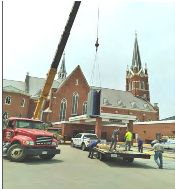
Crews were at work last week installing the new air conditioning system for the church.
